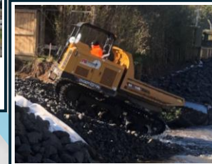
SMALL CATERPILLAR TRACKED MAROOKA CRAWLER WILL LIFT AND CARRY ROCKS TO EXCAVATOR
