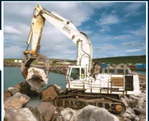
CATERPILLAR TRACKED EXCAVATORS CARRYING ROCKS TO BEACH ACROSS COMPACTED GRASS TO SAND
