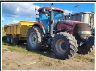
PNEUMATIC WHEELED TRACTOR AND TRAILER DELIVER ROCKS TO THE BEACH FRONT WORK AREA
