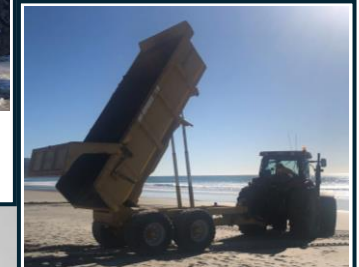
TRACTOR/TIPULATOR UNLOADS ROCKS DOWN 1.5m ONTO SAND. LOCATION VARIES WITH WORKS THROUGH THE DASHED AREA.
