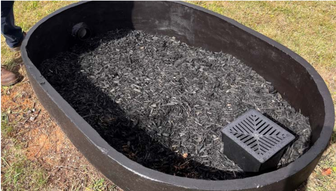
Figure 8: Non-compliant raingarden with no vegetation
