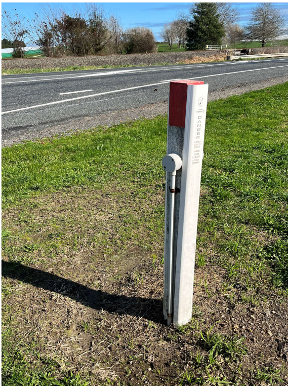
Figure 5.5 Marker identifying buried cables at the intersection of SH2 and Arawa Road
