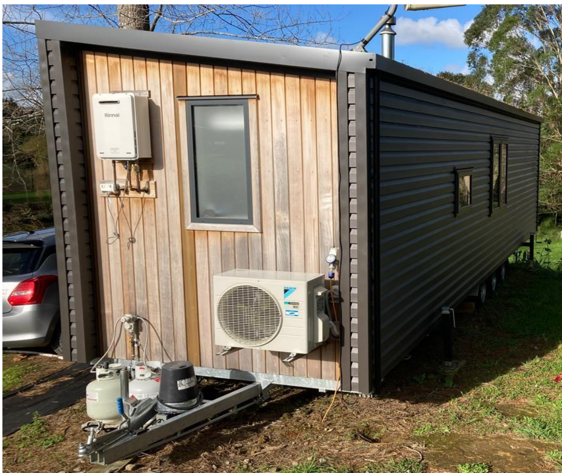
Example above of other systems/services (heat pumps) connected to the unit only
