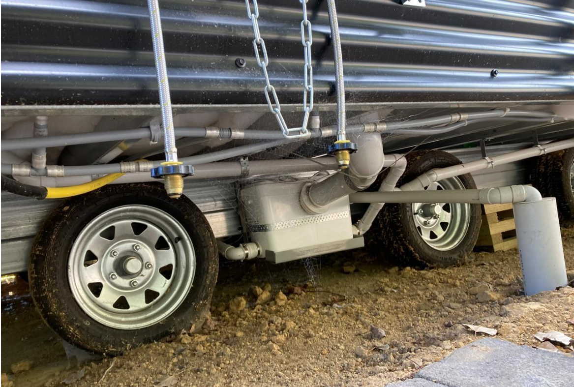
Example above of waste pipes that are not easily disconnected
