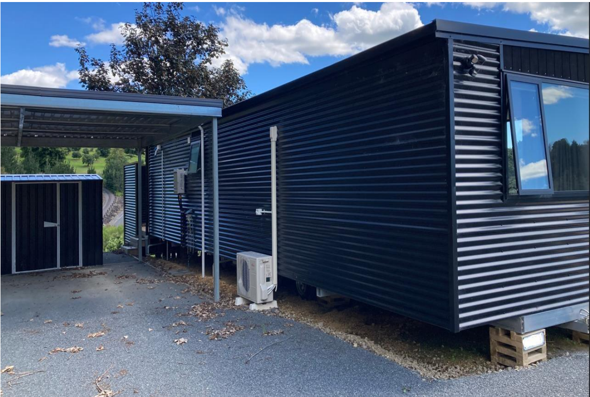
Example above of other systems/services (heat pumps) that are connected to the ground
