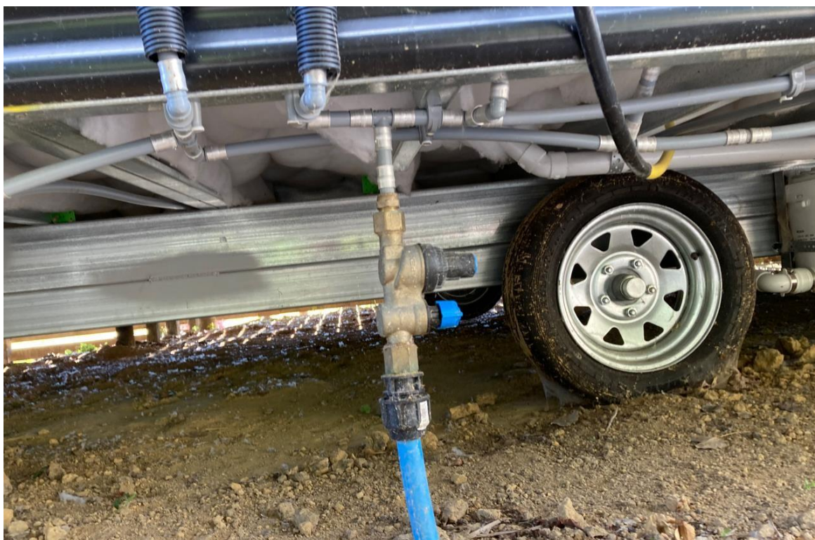
Example of a water connection that can be easily isolated and disconnected
