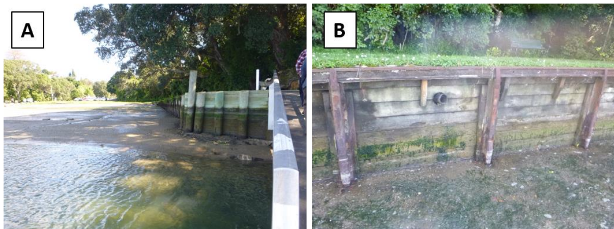
Figure 2-3 Examples of protection structures around Tanners Point. (A) Timber seawall and pontoon (Cell 2F), (B) timber seawall at the edge of grass reserve (Cell 2F).
