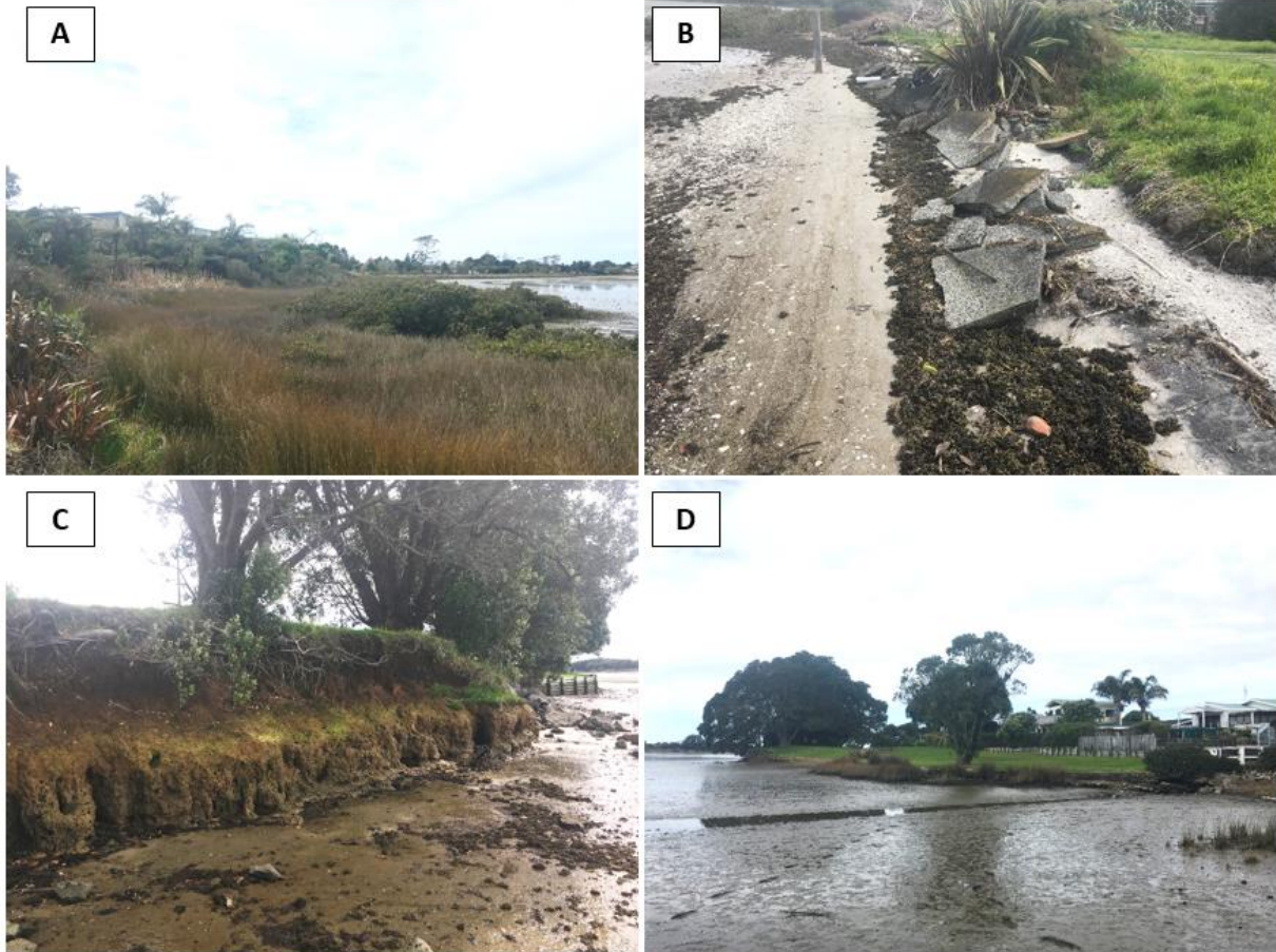
Figure 32-2 Site photos for Athenree. (A) Low-lying estuarine shoreline within Cell 32A. (B) Sandy high-tide beach (Cell 32C). (C) Consolidated bank (Cell 32E). (D) Sheltered, consolidated bank (Cell 32G).
