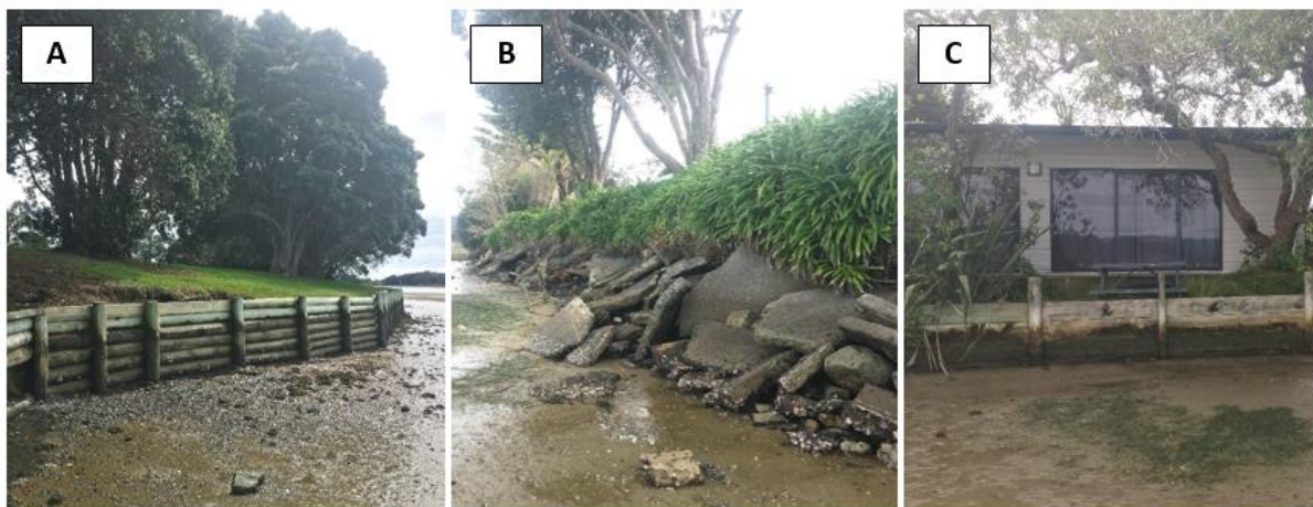
Figure 32-3 Examples of protection structures along the Athenree shoreline. (A) Timber seawall (Cell 32E), (B) section of riprap (Cell 32E), (C) timber seawall (Cell 32E)
