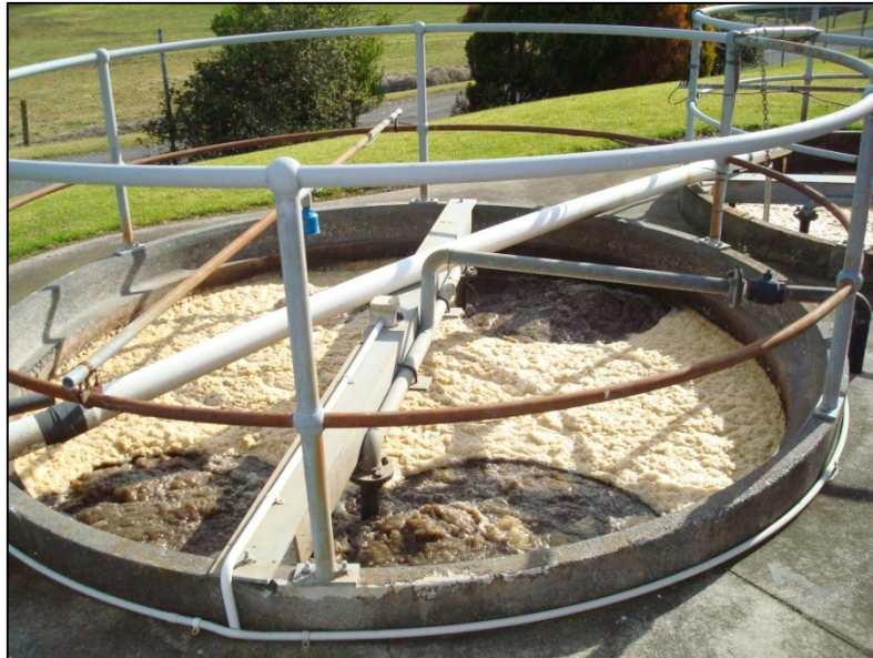
Figure 5 Sludge Storage Tanks
